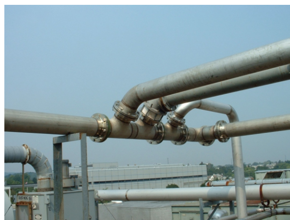
Coated Schedule 10 vent pipe installed on the roof of a Pennsylvania Specialty Chemical plant, replaced leaking Schedule 40 stainless steel pipe. Vent streams are from glass-lined steel and Hastelloy reactors and centrifuges. ( Photo courtesy of J. Brobson, Design Plastic Systems, Inc. )
