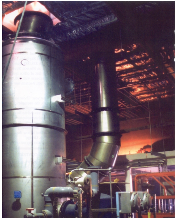
Coated duct connected to scrubber unit at a California Biopharmaceutical pilot plant. Building was completely renovated from warehouse to cleanroom research facility use. ( Photo courtesy of G. Cortes, SMW 104 )
