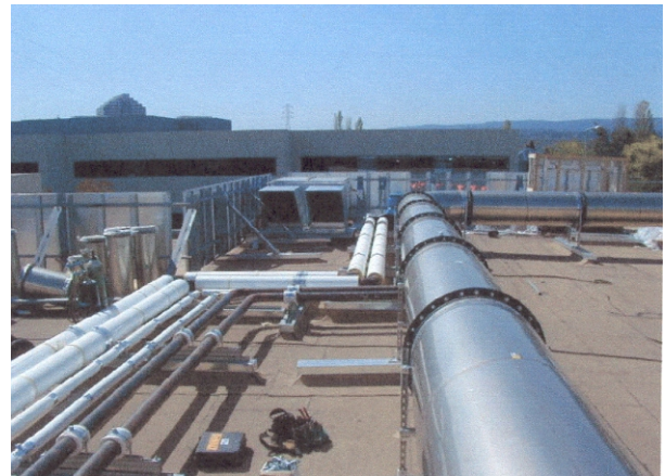
Coated duct installation on the roof of a California Biopharmaceutical Pilot Plant. ( Photo courtesy of Hellwig Plumbing )
