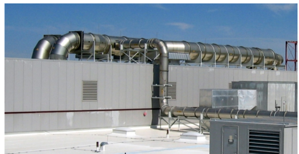
First used in the semiconductor market, coated stainless steel duct has gained acceptance in numerous other industries. No UV or external coating is necessary on 300 series stainless steel. ( Photo courtesy of Fab-Tech, Inc. )
