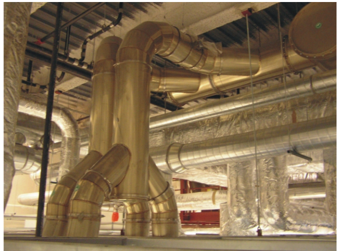
Interstitial level of Weaver Lake 3 facility with PSP® duct shown in the foreground with connection to horizontal header.
